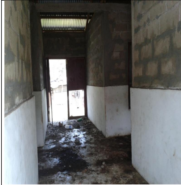
Picture 3 Condition of toilet in Taibesi market
