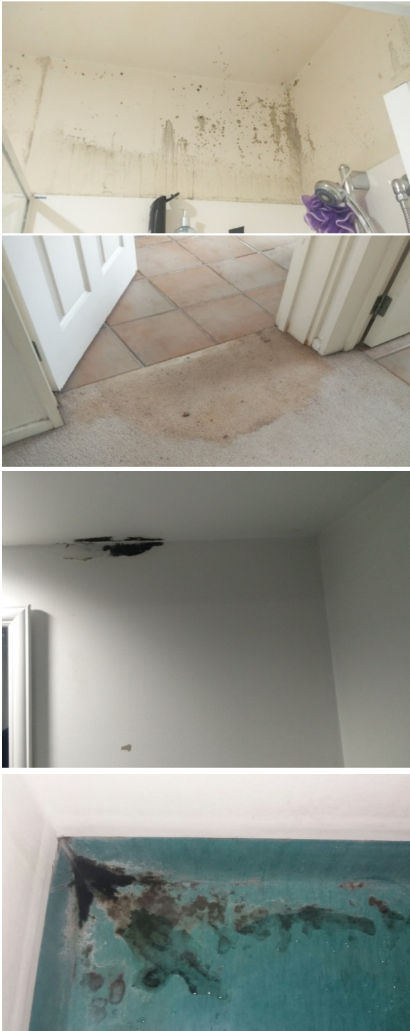
Figure 5: Indication of mold growth and dampness on walls/floor found in some of the participants' households
