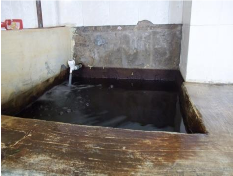
Figure 22: Sink with stagnant water
