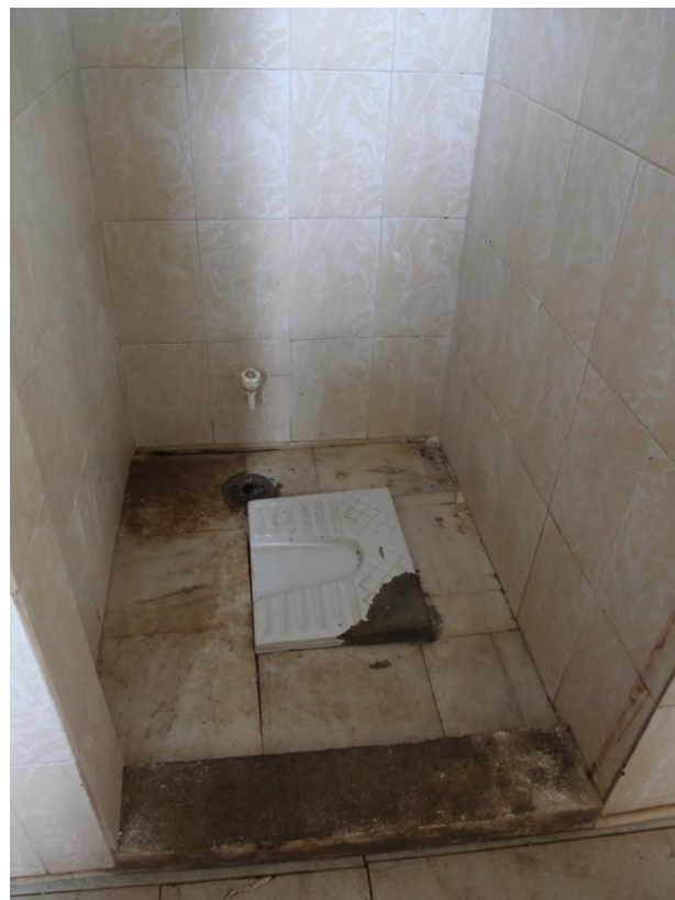
Figure 28: Broken squat toilet
