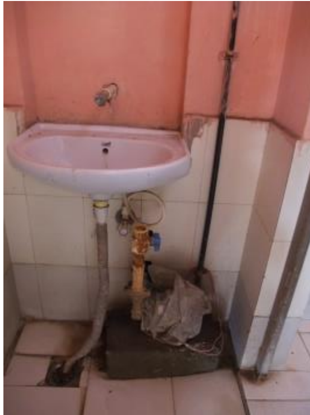
Figure 29: Broken basin in a toilet block
