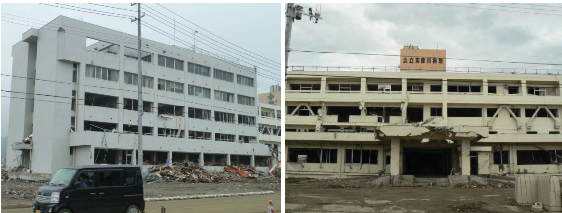
Figure 57 Shizugawa Hospital (west building) – the taller of the 2 hospital buildings at 5-storeys, this section suffered less debris damage than the east building.
