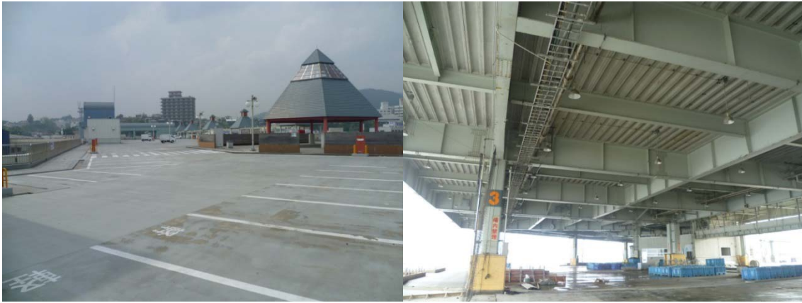
Figure 49 The large open car park roof space above the fish market provided refuge to 1000 people. This structure is at the harbour front and inundation almost reached roof level. The open steel structure enabled tsunami flow at the 1 st storey.
