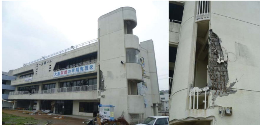
Figure 46 An office building in the inner harbour was unused on March 11 th . This building sustained debris damage to the external stairs (front right) which face the harbour. Minor scour occurred along the seaward face of the building, and around the base of the external stairs.
