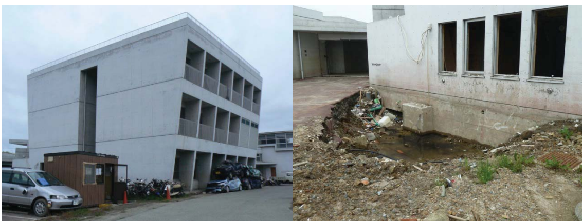
Figure 48 An elderly persons' welfare centre which was inundated to around 8 m height. Scour up to 2 m deep occurred on the near side of the building in this photograph. Extensive damage occurred immediately inland of this building, while 80 survived on the upper floors.
