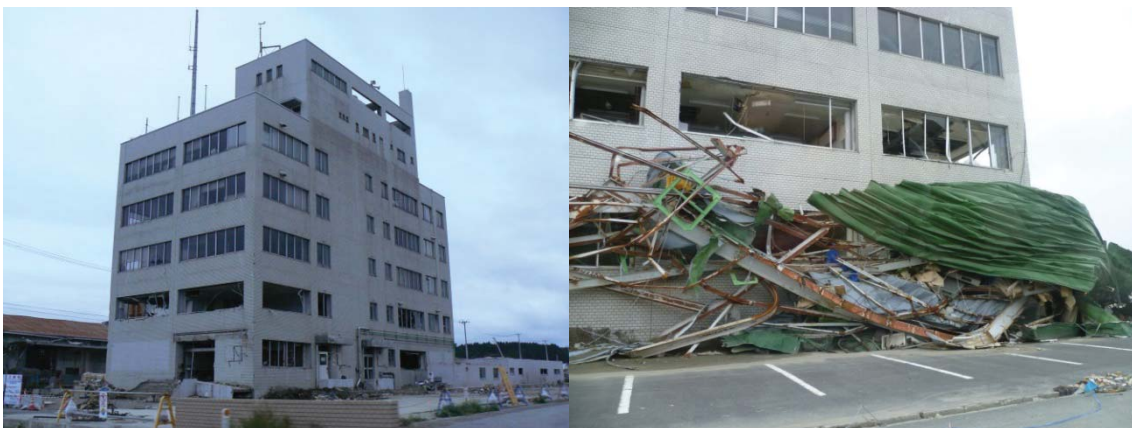
Figure 51 The National Government office, where 120 people took refuge from the tsunami. This building is adjacent to the Prefectural Government offices and was left undamaged when light steel structures were washed into it. The lower two storeys were inundated.
