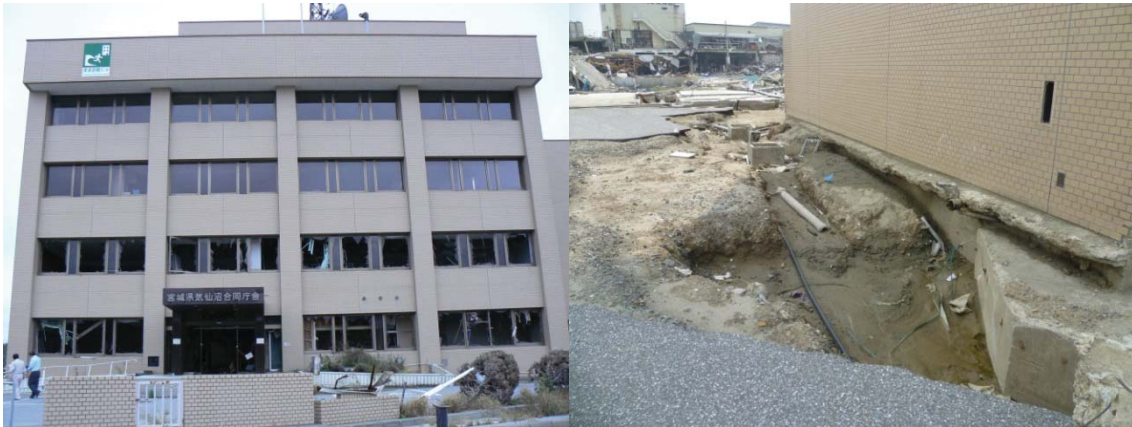
Figure 50 The Prefectural Government offices suffered extensive scour and heavy inundation of 8 m. This building was constructed after 2004 and displays tsunami vertical evacuation signage at roof level. 200 people survived the tsunami in this building
