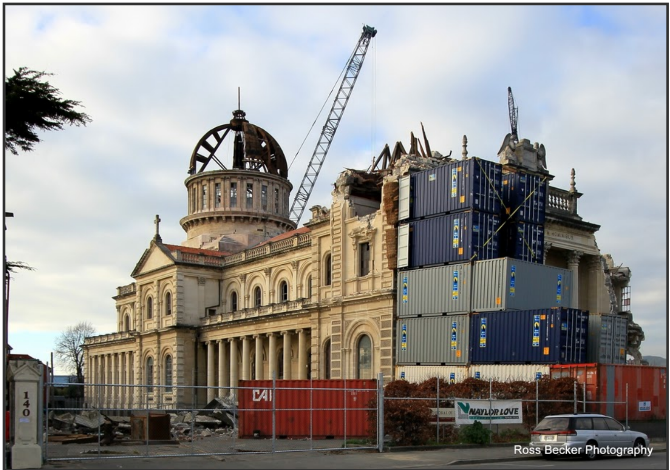
▲ Basilica of the Blessed Sacrament, with damage ‘contained’, September 2011 — ©2011 Ross Becker
