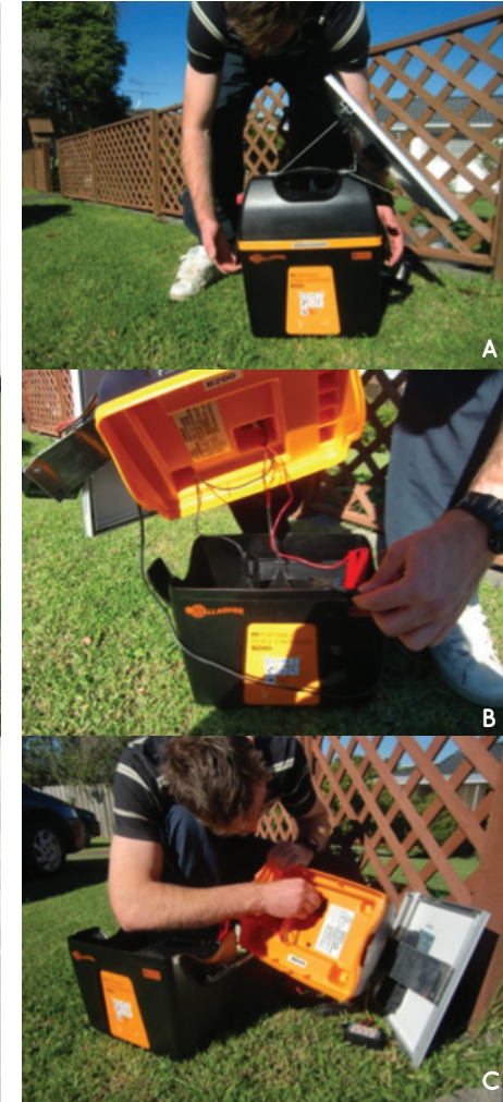
Figure 28. A) Opening Gallagher B100 to investigate the inside components. B) Placing lid back after hooking crocodile clips from energizer to battery terminals. C) Checking connections to identify where the problem lies
