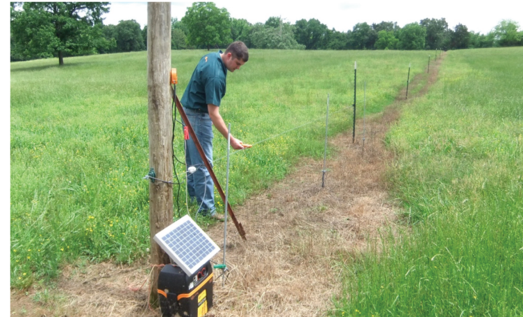
Figure 25 - Evan measuring 5.6 kV on the single wire fence powered by the B100SP (running full power).
