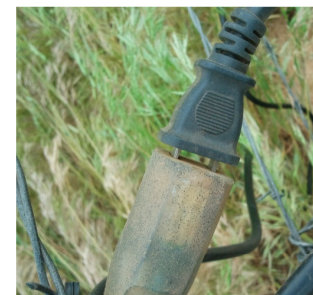
Figure 12 - The M300 mains cable plugged into an extension cord and exposed to the elements.
