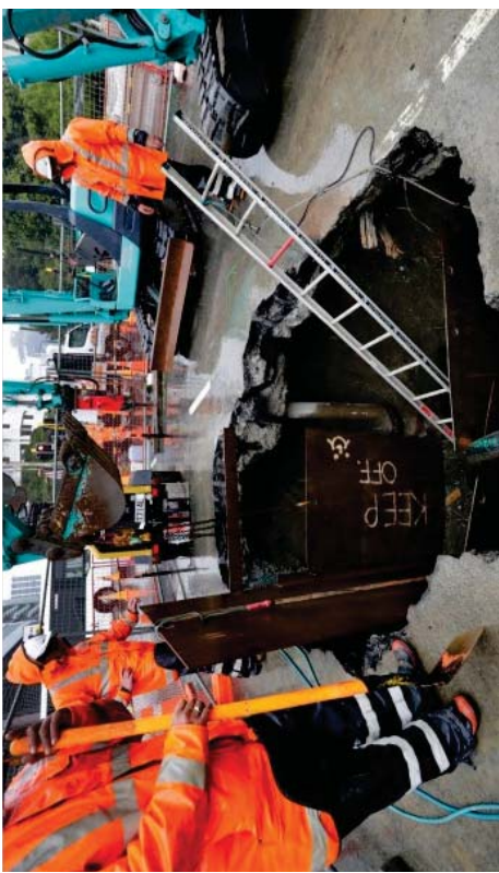
Fig. 9. Featherston Street sinkhole.
