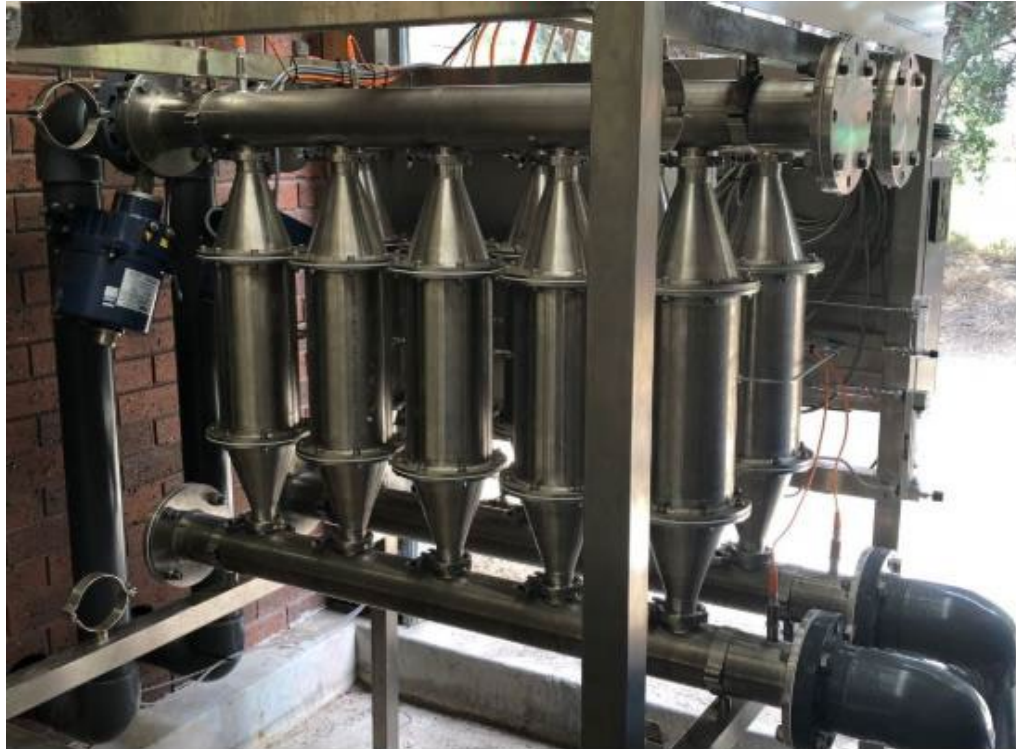
Figure 6. Example of a multiple venturi NB system, using ozone for a golf course turf application, primarily for the elimination of fungal disease, (Nano Bubble Technologies, 2020).
