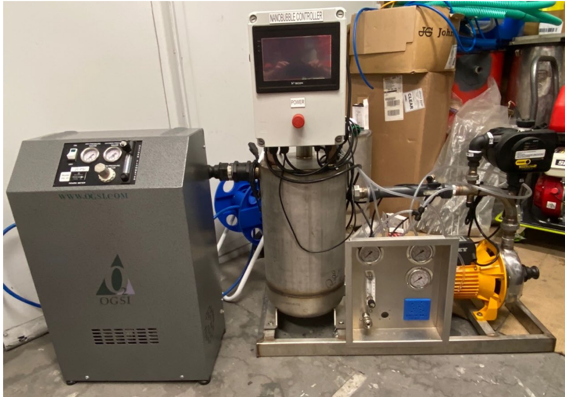
Figure 32 - NBA generator prepared for shipment to Kauri Park. The stand-alone unit at the left of the image is the oxygen generator.
