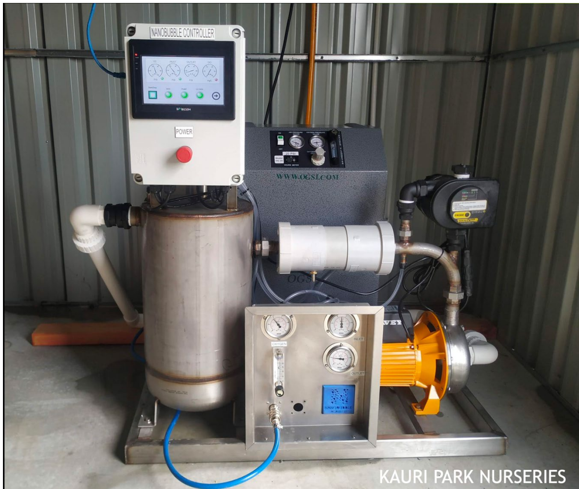
Figure 33 - Nanobubble Agritech generator fully installed and online at Kauri Park
