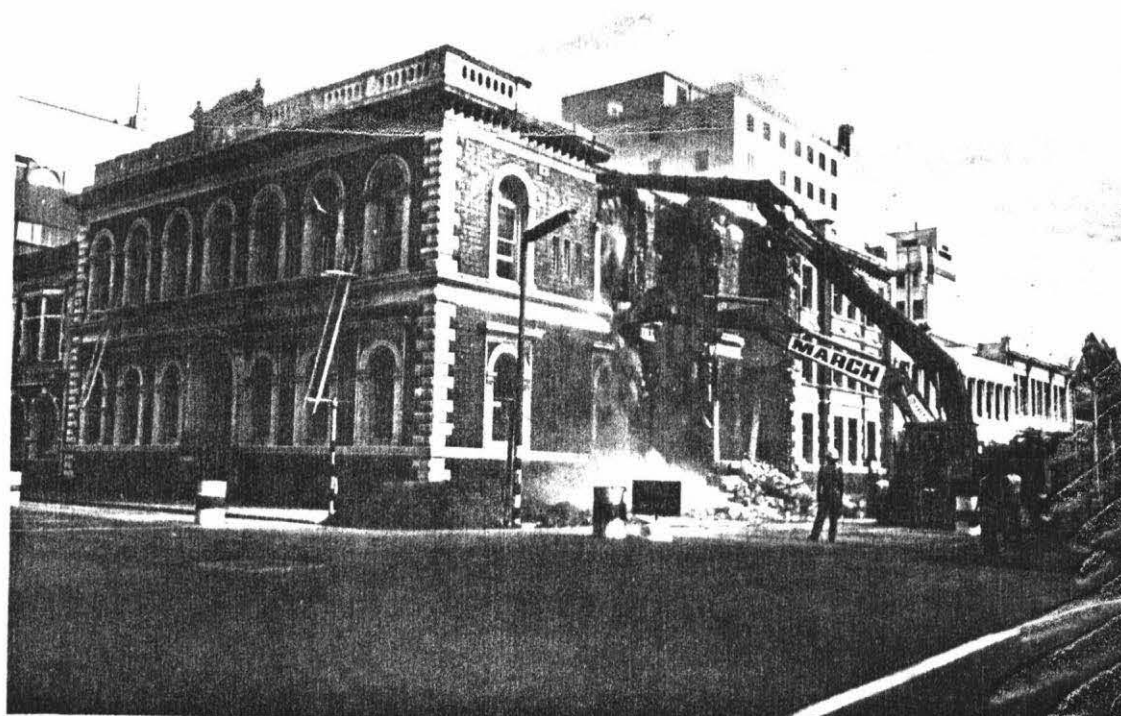
Plate 20 The first blows of demolition to the Old National Bank. (Source: Christchurch Press Co. Ltd.)
