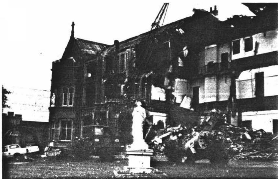
Plate 6 Demolition of the Sacred Heart Convent in December, 1982. (Source: Mr B. Dickson, Architect, Wanganui.)
