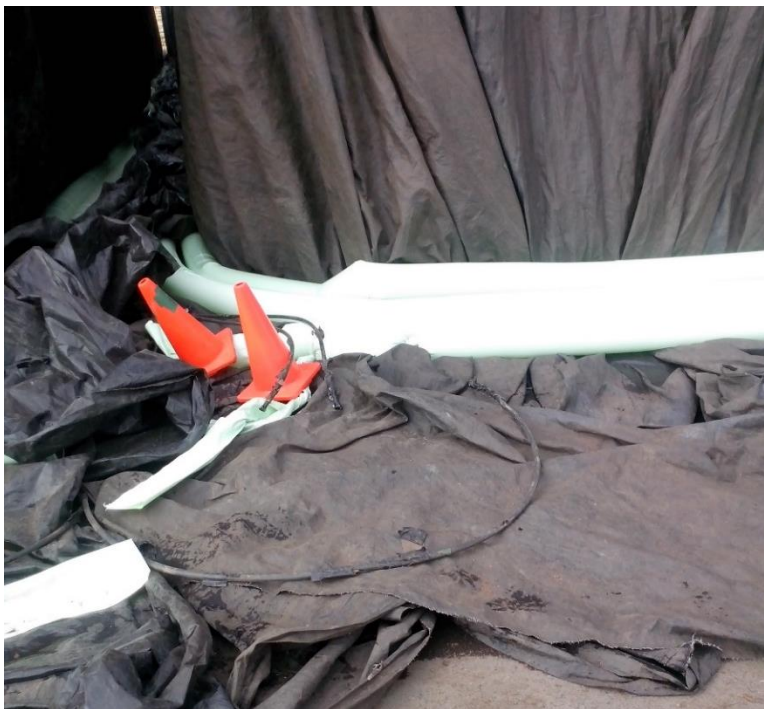
Figure 2.16 Tubing running out of enclosure (R. Hinz)
