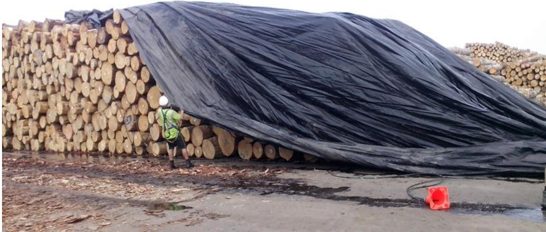
Figure 2.13 Stretching out tarpaulin over log stack. Note methyl bromide introduction tubes and measuring tubes run from the stack to the orange cone (R. Hinz)
