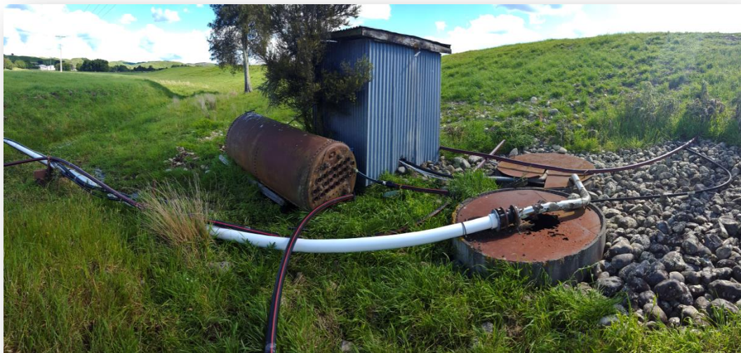
Figure 13: An old style well installed in a productive artesian spring (Kohinui Road, Mangatainoka 40°25'03.8"S 175°52'27.2"E). Large volumes of water were withdrawn from this well to supply the nearby (disused) Dairy Factory.
