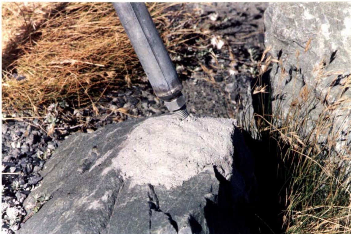
a: Tripod legs concreted onto solid rock.
