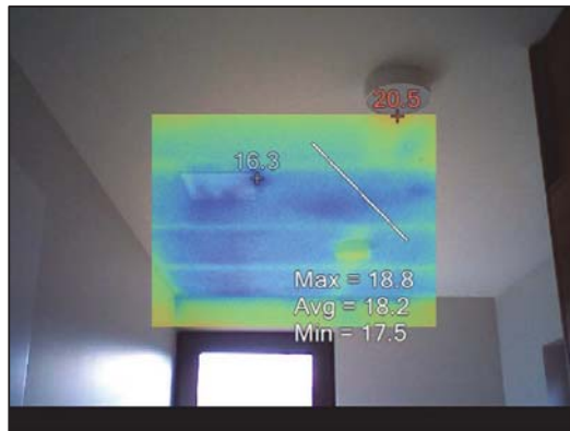
Figure 4.20: A thermograph showing lack of insulation of laundry room's ceilings.
