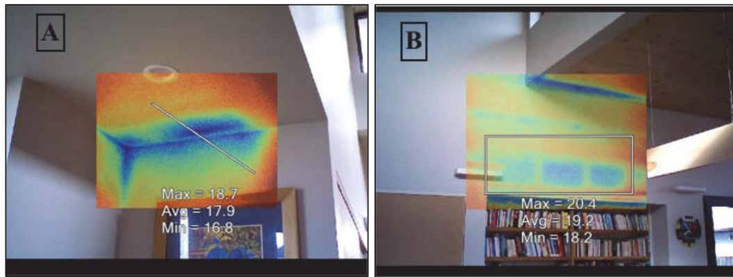
Figure 4.19: Thermographs illustrating lack of insulation (a) at the junction between the wall and the ceiling; and, (b) wall coverage above the bookshelf.
