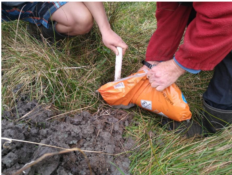
Figure 24: Back filling of an auge hole around the installed piezometer with fine sand around the installed piezometer.
