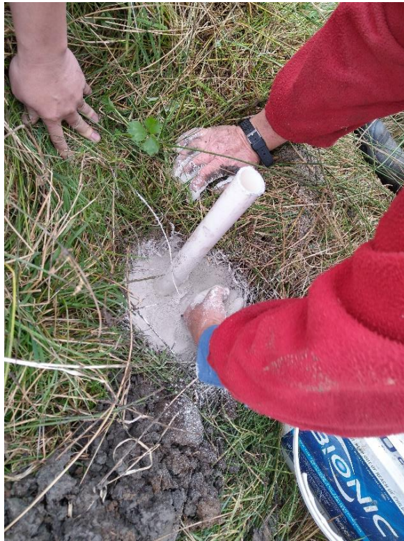
Figure 25: Infilling around the installed piezometer with bentonite clay around the top section of piezometer at surface level.
