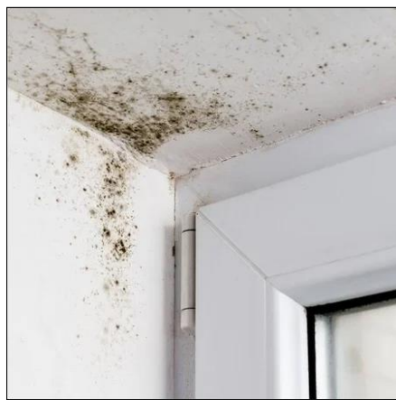
Figure 70. Typical black mould grows with restricted ventilation and elevated humidity due to the condensation and temperature (Twistfix, 2013).
