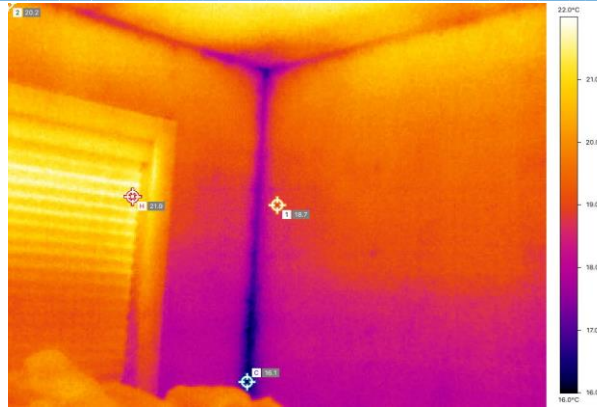
Figure 45. Thermal bridging was created by the corner of the building that has not been insulated (common defect even with 'modern' builds). Source: Author's contribution
