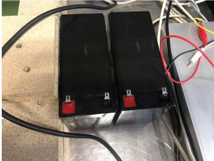
Figure 20 Two rechargeable batteries rated at 12 volts.
