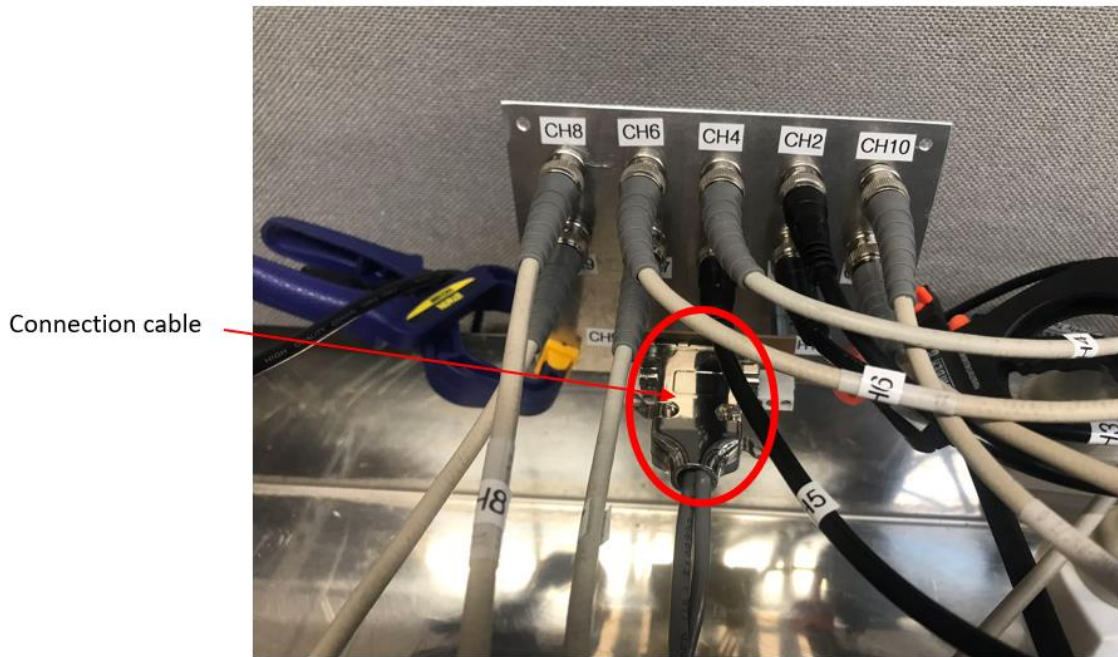
Figure 26 10 Analog output channels connected to a convert plate which has 10 BNC connectors. The transmitting signals will pass to the transmitting array via connection cable.
