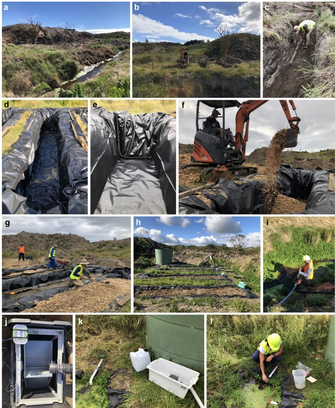
Figure 4.2. Images of experiment installation, procedures, and instrumentation. a) Drain 3 and site selected for the installation of the pilot-scale bioreactors. b) Excavation for the bioreactors. c) Land levelling inside the bioreactor. d) Lining. e) Bioreactor outflow tube. f) Bioreactor filled with woodchips. g) Manual woodchip filling and surface levelling. h) Experimental setup view. i) Water pump installation in Drain 3. j) Tipping bucket. k) Ethanol dosing station. l) Inflow water sampling.
