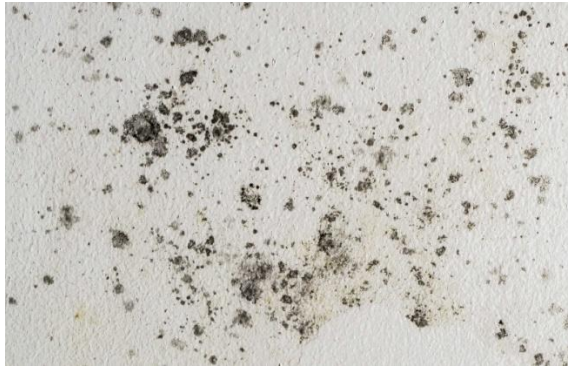
This is a common mold picture that can occur in homes
