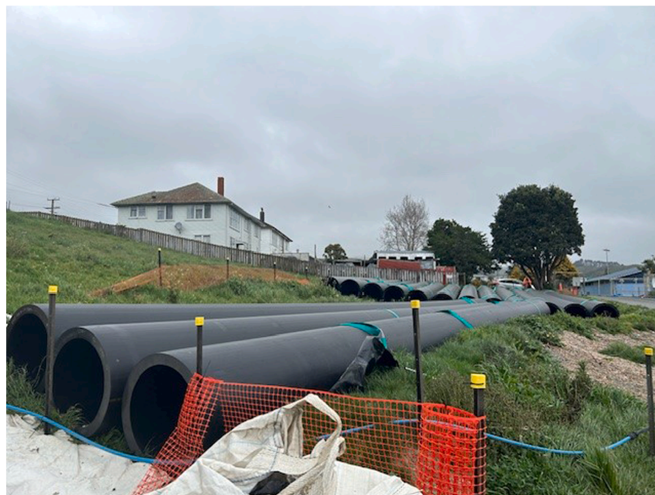
Fig. 6. a A temporary placemaking mini-plaza area; 6b: Materials located on-site for upgrading infrastructure provided by EPR (photos by Crystal Victoria Olin and Philippa Howden-Chapman).
