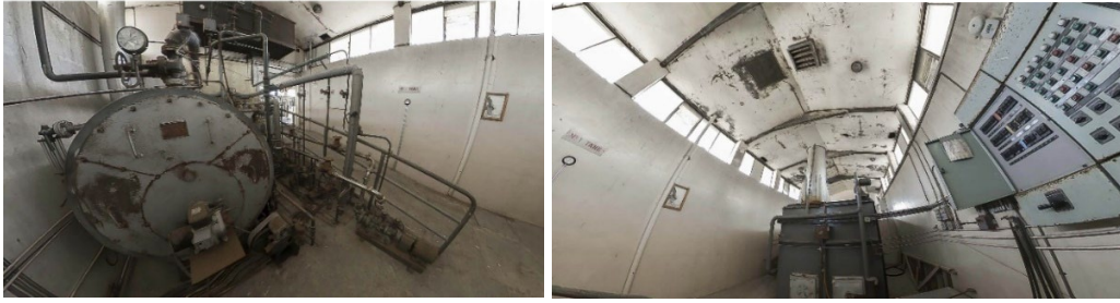
(fig. 109) Doidge, M. (2019). Left. Sterilising tank in boiler room. Right. Furnace and control panel in boiler room [stereoscopic image]. Courtesy the artist.
