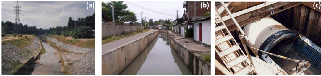
Fig. 5. Structural interventions implemented by SLLDC as flood mitigation measures at Colombo, Sri Lanka (a) St. Sebastian Canal (b) Madiwela East Diversion (c) Pumping station at unity place (Images from Urban Water Center, SLLDC).
