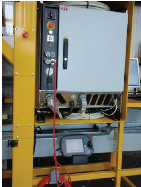
Figure 2.10: Control cabinet to guide the Flex-picker's motion.
