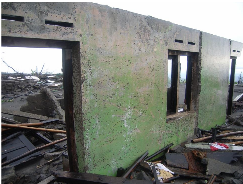
Figure 6.1 Remaining flow parallel wall in Kaliadem. The remains of a house in Kaliadem show almost complete destruction. Only a wall that stood parallel to the flow direction remains after the passage of a pyroclastic density current. Due to the orientation of the wall, the dusty gas pressure only acted on a small area. The wall still shows signs of pockmarks. Photo courtesy of Gert Lube.
