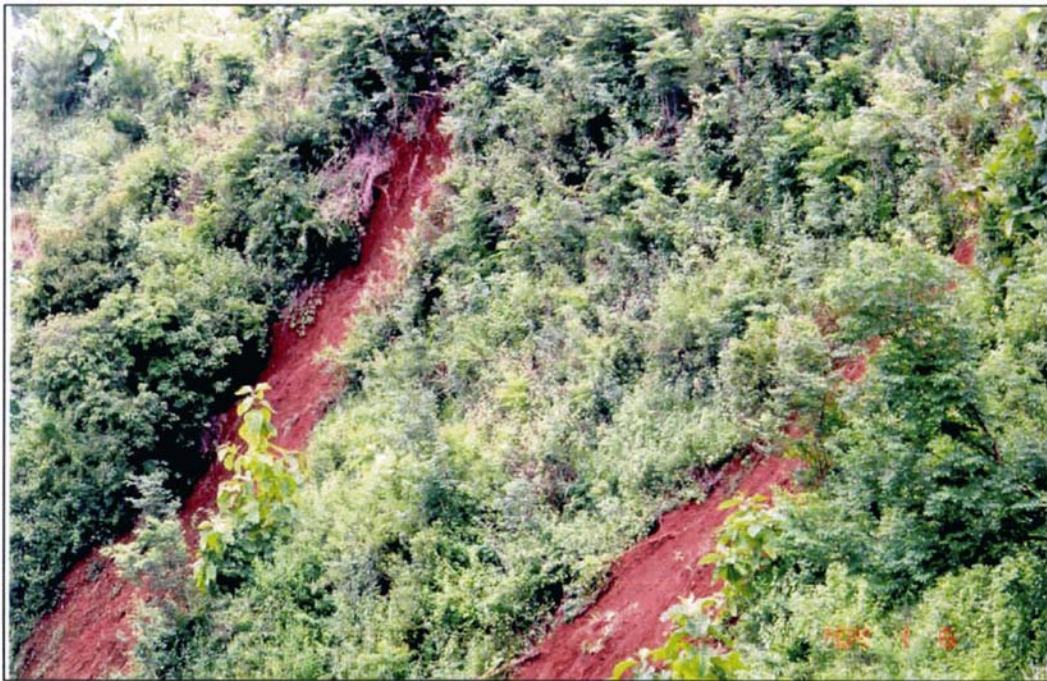
Figure 2-19 Erosion on a dry, steep slope
