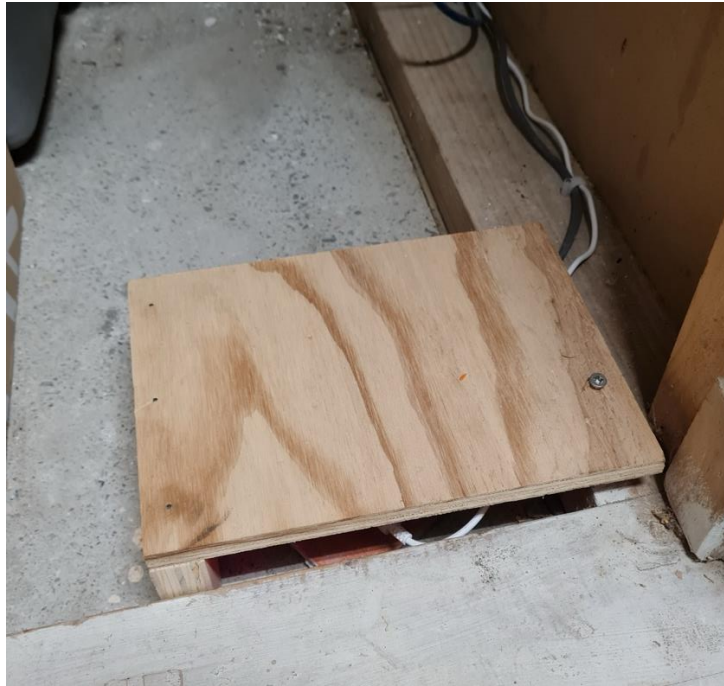
Figure H-5. Sensor installed on a concrete floor in a storeroom, aligned to true north, and secured with a wooden box to avoid disturbances.
