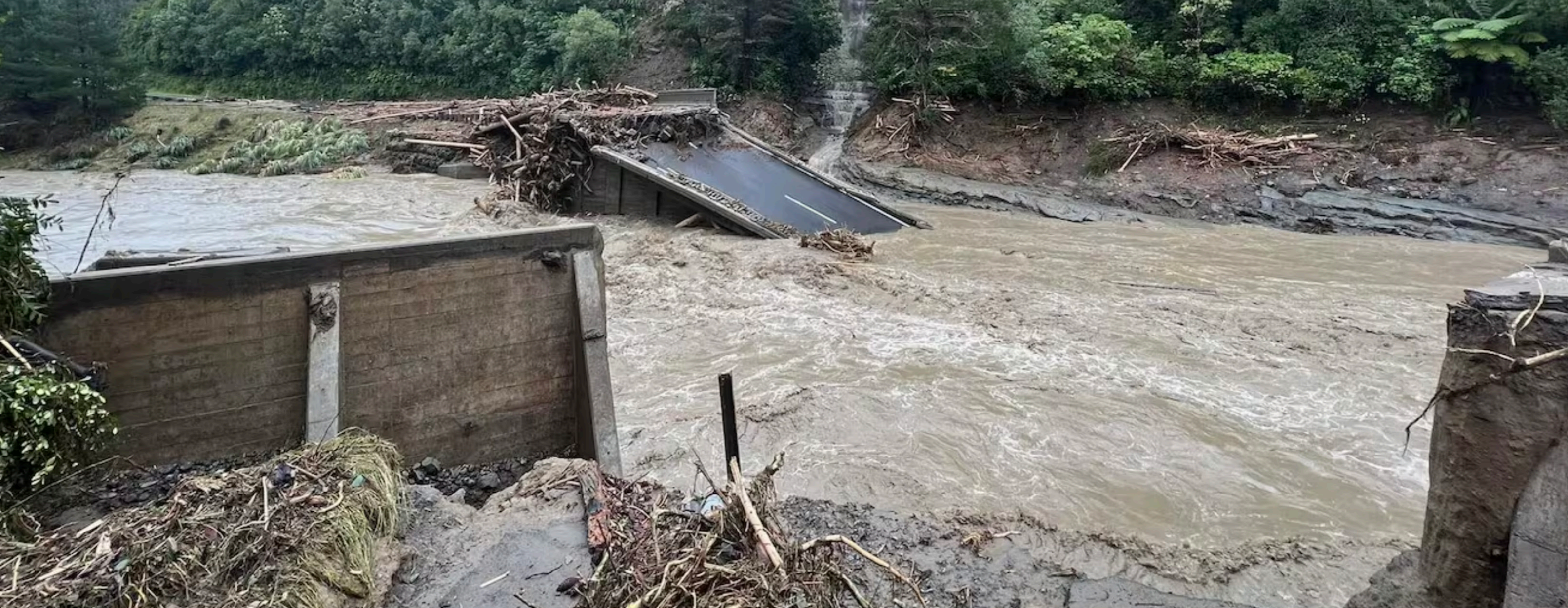
Fig. 3. The Waikare River Bridge near Putorino collapsed in wild floodwaters caused by Cyclone Gabrielle Tong, Rosie. 2023.
