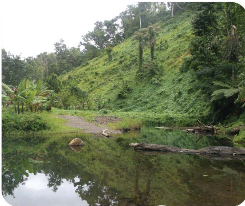
Figure 19. 70° steep slope of an abandon agricultural land on the western side of STN6
