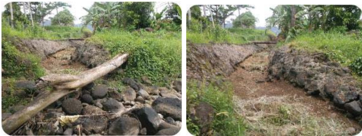
Figure 40. Road drainage as pathway of stormwater from the main road of Tuana'imato into the river
