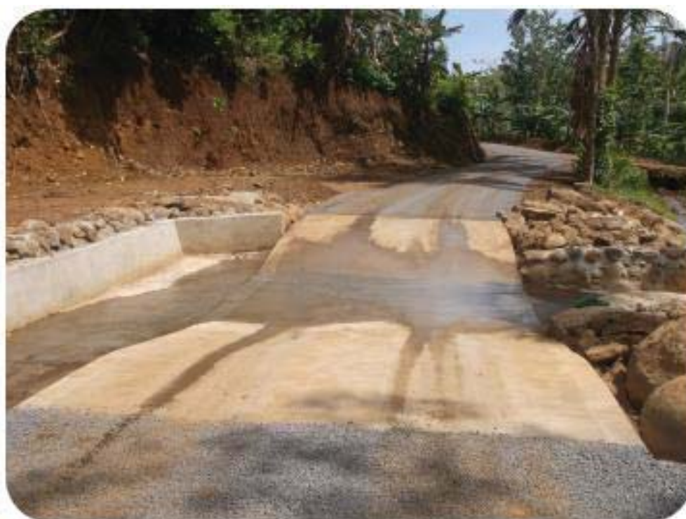
Figure 43. A road ford & eastern view to the newly built road accessing the SWA water intakes
