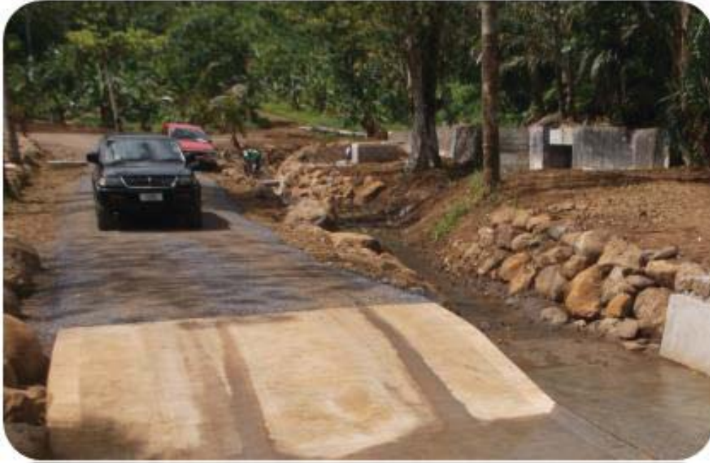
Figure 44. Newly built-road to Chinese 1 & Chinese 2 SWA water intakes upstream Also shows the newly constructed stream path (i.e. diversion) from the river's usual path.
