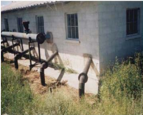
Image 7: Pump House at Bonde
