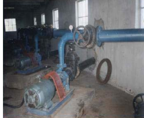
Image 8: Pumping Unit at Bonde
