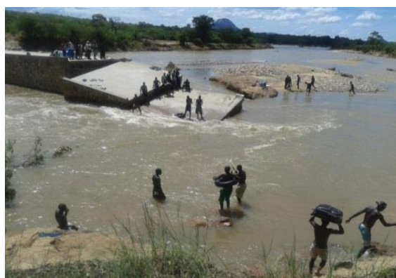
Image 11: Washed away bridge at Rwenya River, pre-field work visit, December 2012
