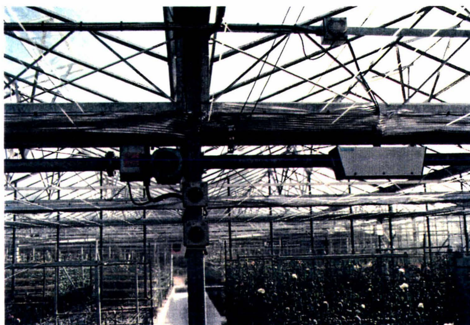
Plate 2.3 Reversible electric motor, torque tube, and cable support system.
