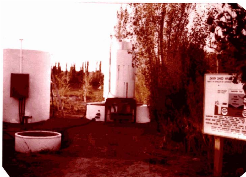
PLATE 5:3 Anaerobic tank and trickling filter arrangement for field plant.
