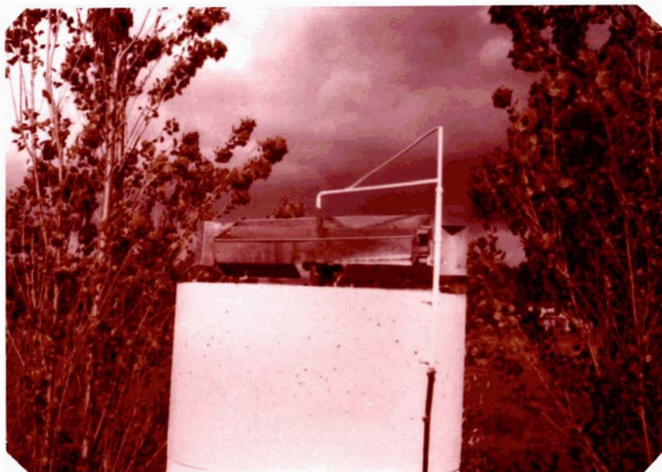
PLATE 5:5 Rotary tipping bucket distributor on top of the field plant trickling filter.
