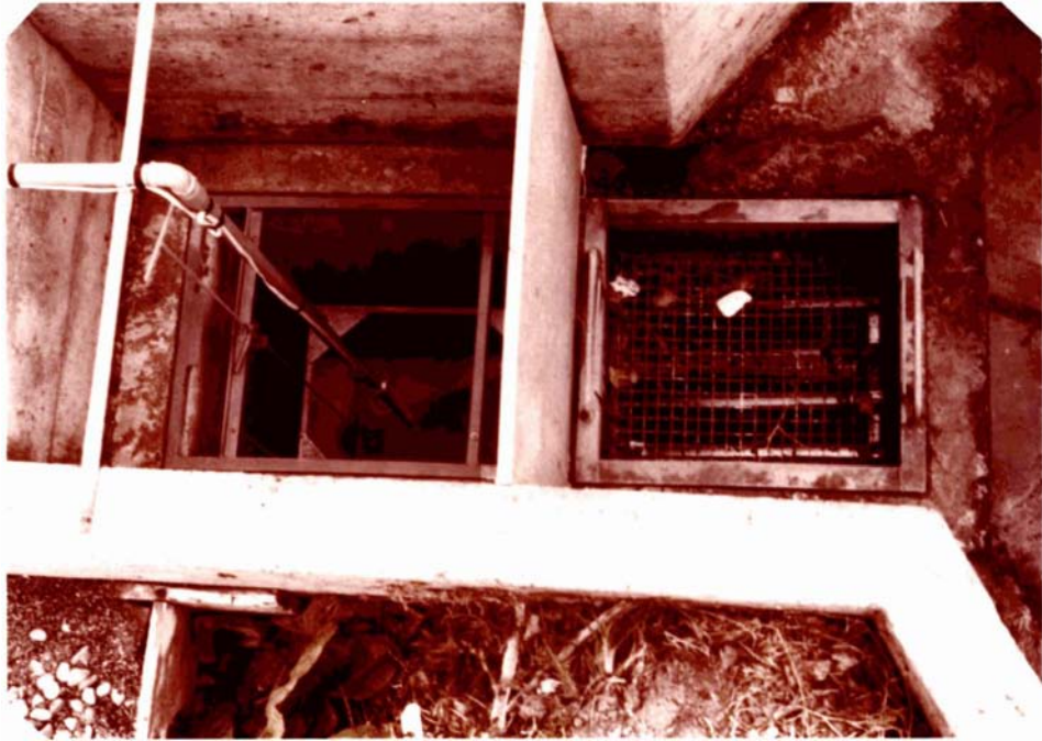
PLATE 6:1 Effluent collector showing the collecting channels (below basket) and the collecting tank. The cable on the outlet pipe is for pump probe control.
