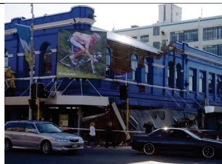
Photo: Cycle Building damaged on 4 September 2010. Retrieved from: http://www.ceismic.org.nz/search/33695937
