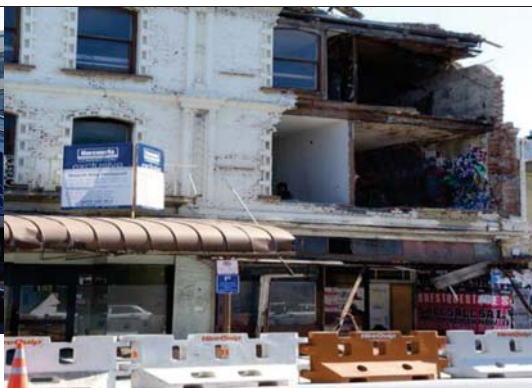
Photo: Building damage from 04 September 2010. Retrieved from: http://www.ceismic.org.nz/search/33695916
