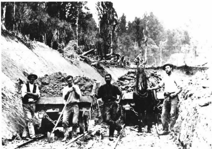
PLATE 9 - Cutting on Main Trunk, 1880's: many towns on the main trunk had boom periods during the period of railway construction and many construction workers later applied for land in the area.
