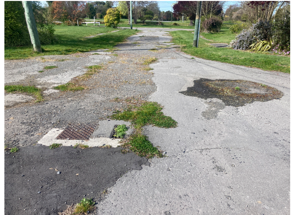
† Fig. 11. Patchworked road in the residential redzone, Richmond, Christchurch, 2022
