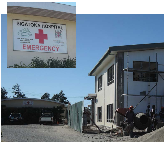
Photograph 7.2. Sigatoka Hospital, with the new maternity unit under construction in the foreground.
