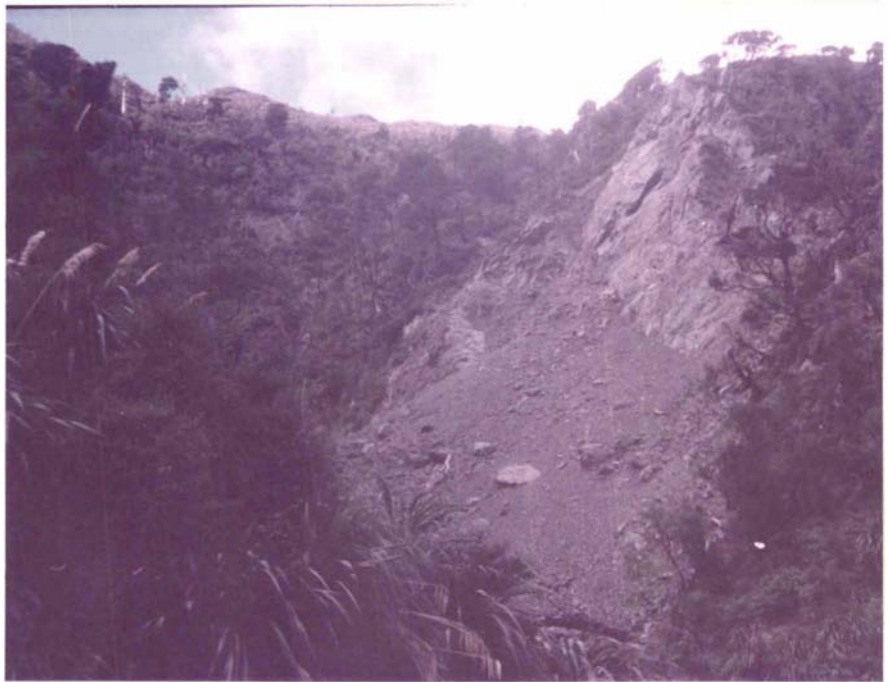
FIGURE 10.11: Rock fall resulting from failure along the north-south trending joint system. The planar joint surfaces dip steeply towards the west (left). Channel at base of rock fall is choked with coarse angular rock fall detritus. Photograph taken in North Oruakeretaki catchment at T23/593091.
