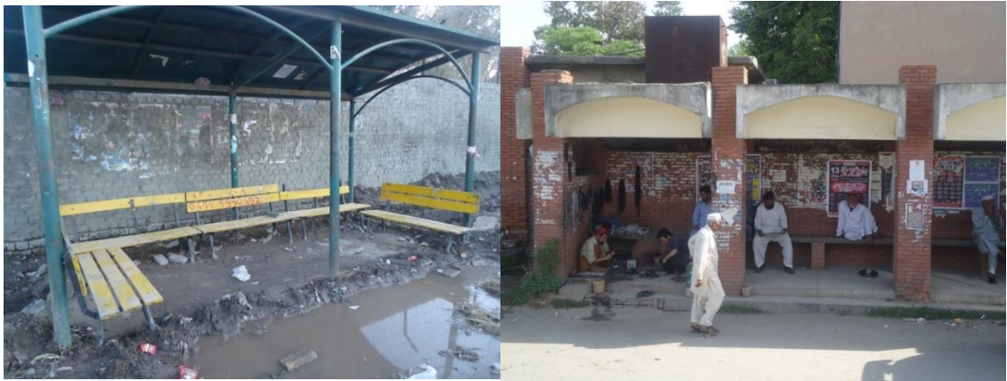
Figure 7. 11: Condition of bus/van stops in Rawalpindi
