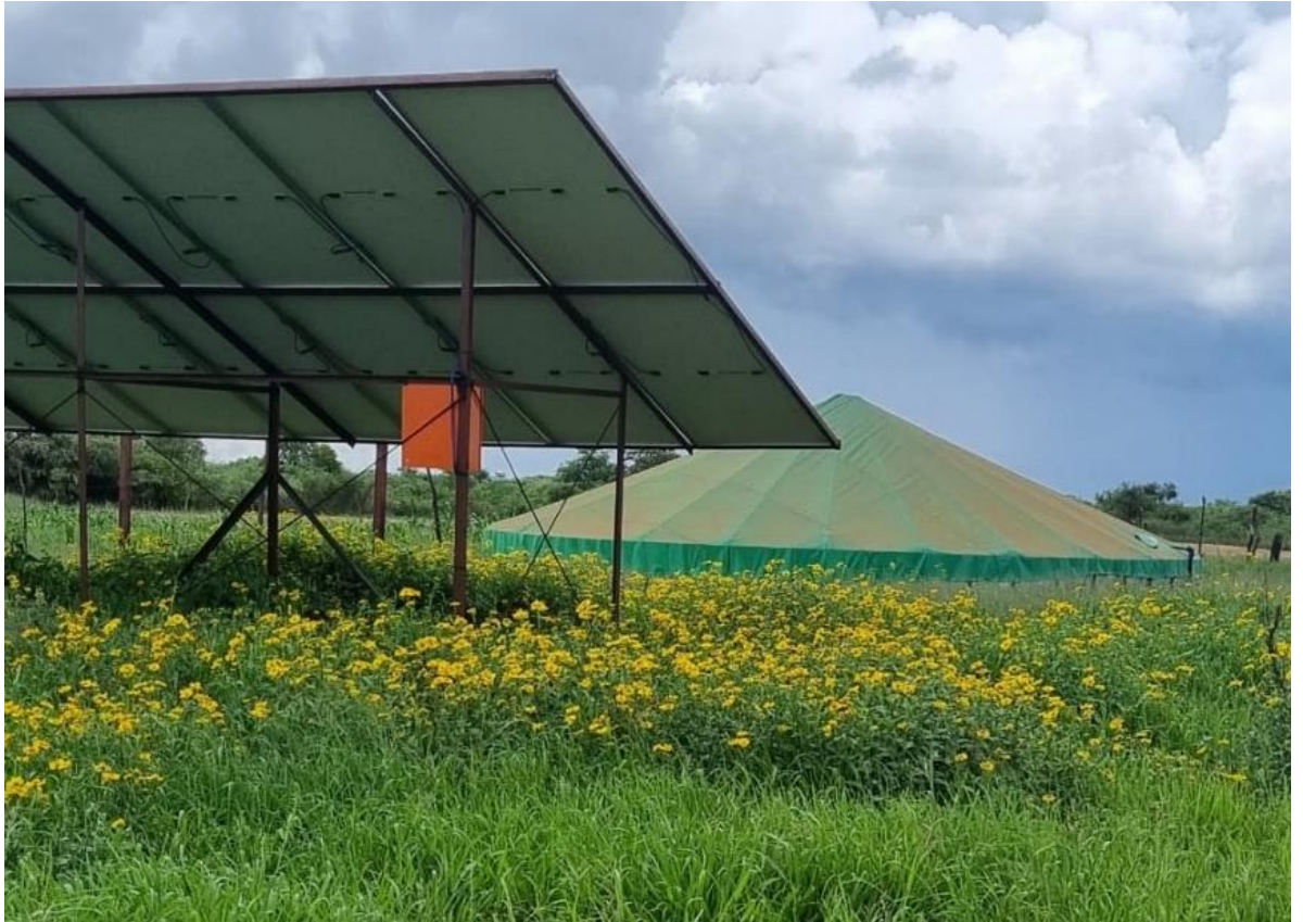
Figure 7: Solar panels for the borehole pump and reservoir purchased under IAS
