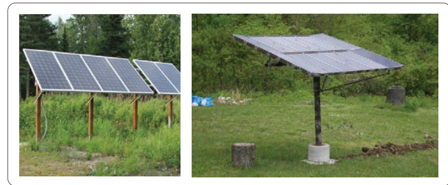
Figure 25. Stand alone solar array frames (Bowie, 2009).
