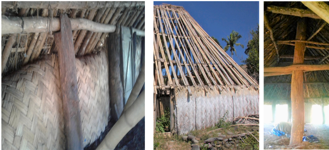
Fig. 18. Interlocking connection (left), lashed connection between rafters and purlins (middle), central post connection (right).
