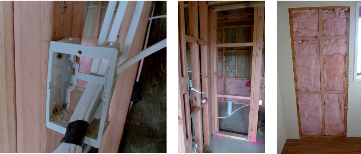
Figures 97-101 – Balloon Framing, Plasterboard and what lies beneath, by Author, courtesy Simon Wain, Torbay.
