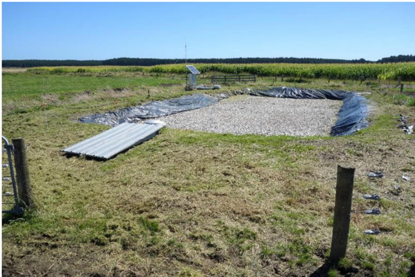
Figure 3. Waitatapia denitrification bed prior to soil covering (February 2021), (R. Gray, Massey University).
