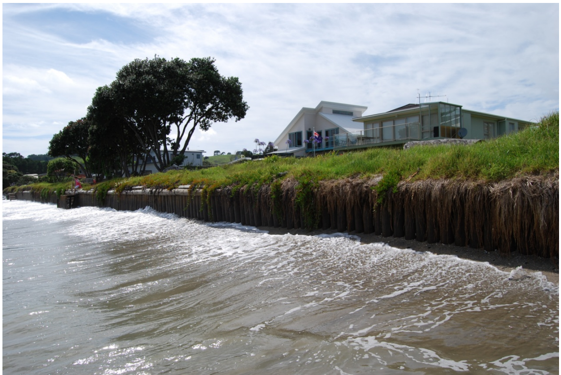
Figure 6.17: An example of public interests going ‘out the window’: this section of Cooks Beach is experiencing an entire loss of public lateral beach access due to shoreline armouring to protect private beachfront property (photo by author, 2012).
