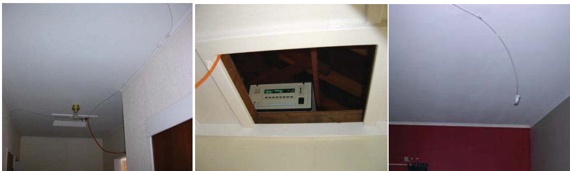
Fluorinated ethylene propylene tubes to draw the sampled gas from each room to the nitrogen oxides analyser located in the roof cavity.
