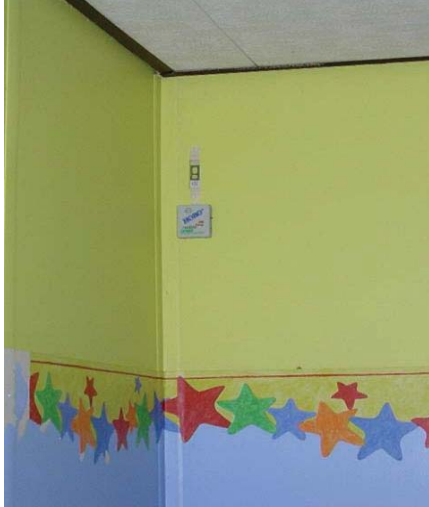
Figure 3.7: Typical sensors location on the inside surface of an external wall: fungal detector (top), temperature/RH Hobo ® logger (bottom).
