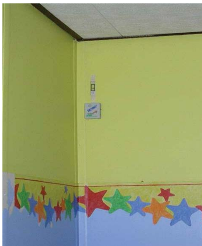
Fungal detector (top), temperature /RH logger (bottom) on the inside surface of an external wall
