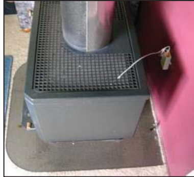
Thermocouple connected to a wood stove
