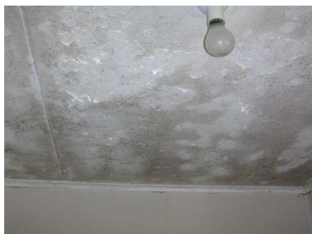
Mould and damage to a ceiling
