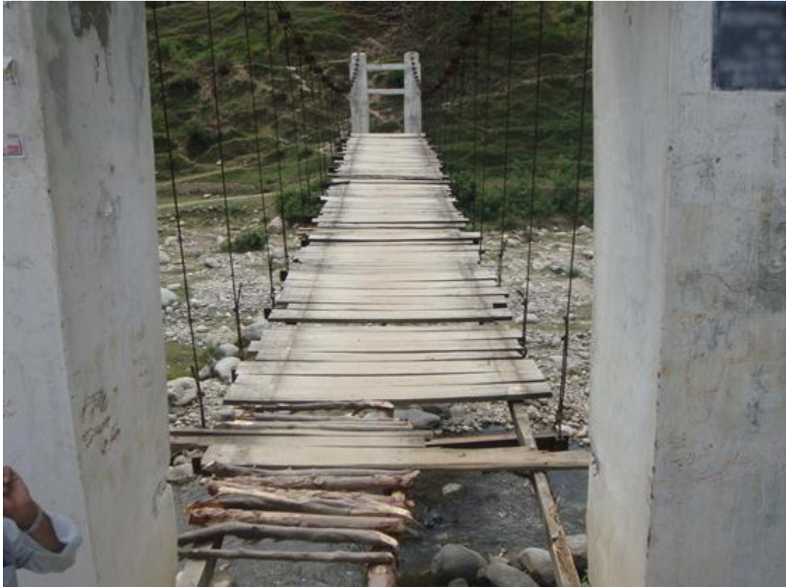
Figure 4-2: The dilapidated bridge in Banda-1, the only access to the village
