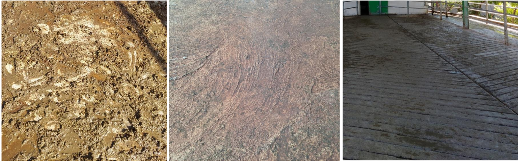
Figure 2. Different surface quality scores in parlour holding area—(Left) Score 1: a smooth surface with potential chance of slipping; (Middle): Score 2; non-grooved surface, but rough enough to reduce slipping; (Right): Score 3; grooved concrete or rubber mats where chances of slipping are low.
