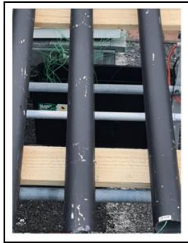
Figure 9-5 Coating removal and degradation of Tubes
