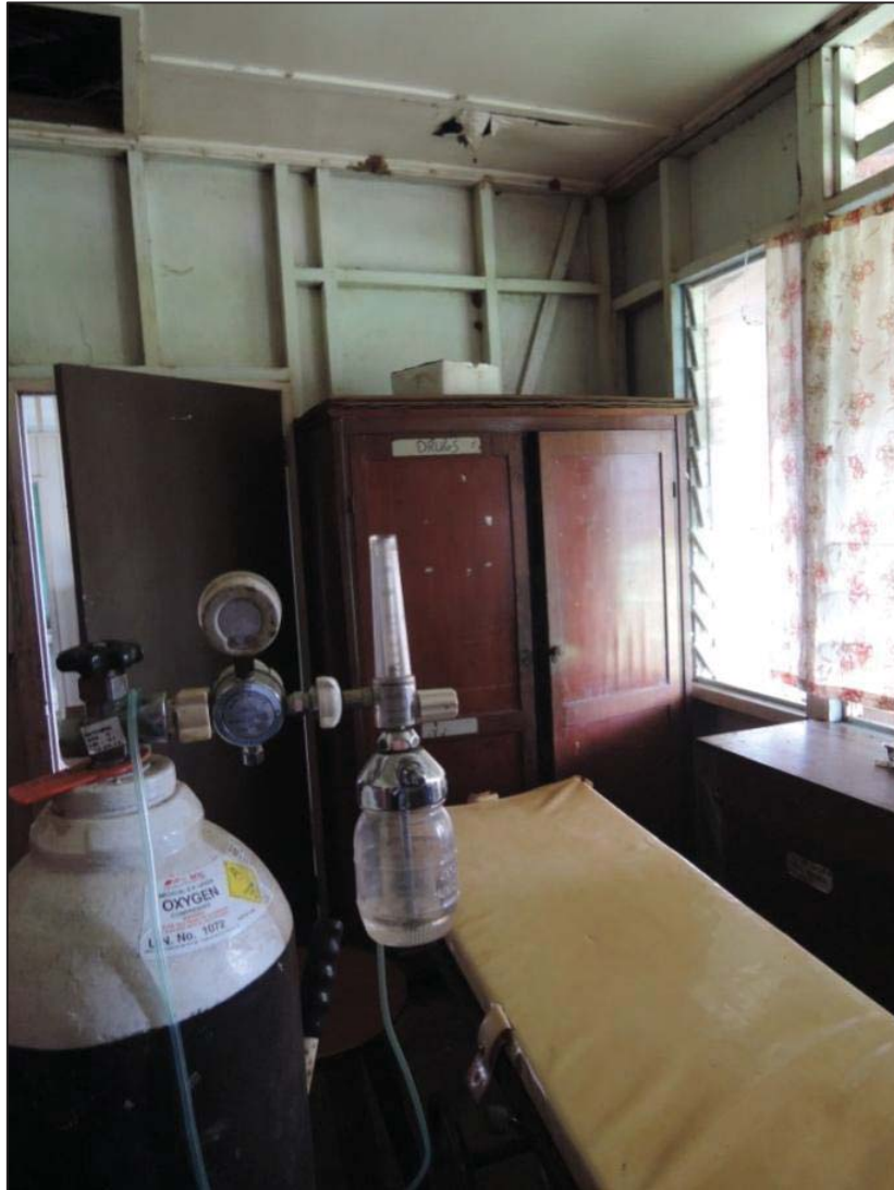
Photo 6: The Emergency Room in Palie Health Centre (October 2014). As evident within this photo, the ceiling of the hospital is now rotten in many places.
